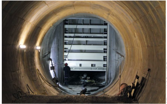
Figure 8: Replacement of the hydraulic steel facilities, upper sluice gate in the bottom outlet
