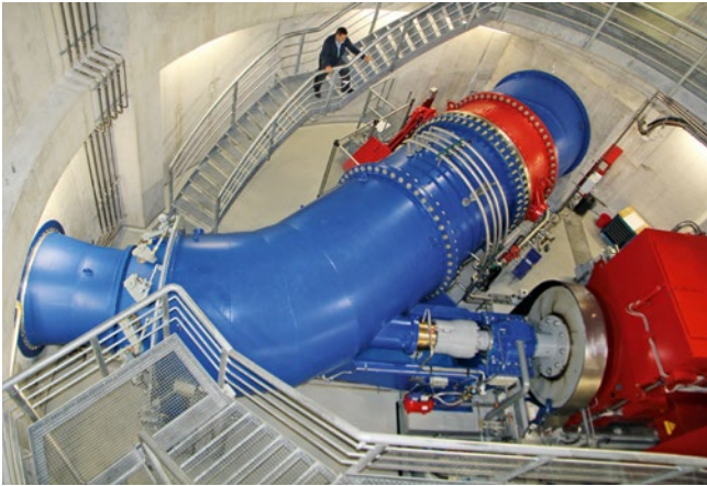
Figure 7: Compact axial turbine at hydropower station II
