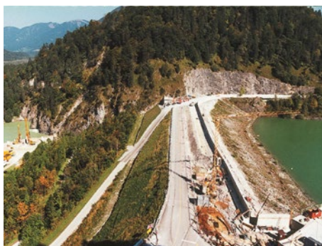
Figure 5: Construction of the crest wall and banking for the elevated section of the dam
